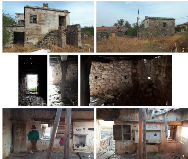
Figure 10. Photos of the house in parcel 1497. 1. West façade, lime plastered surface, exterior stair, slate stone eave, chimney. 2. South façade, partially plastered surface, slate stone eaves. 3. Entrance of the barn. 4. Post, main beam, and secondary beams of the barn. 5. Unplastered wall surface of the barn, niches. 6. Bathing cabinet ( yunak ), window, shelf, post, and niche for water jug in the living space. 7. Door, cupboard, match niche, fireplace, post, window in the living space.
