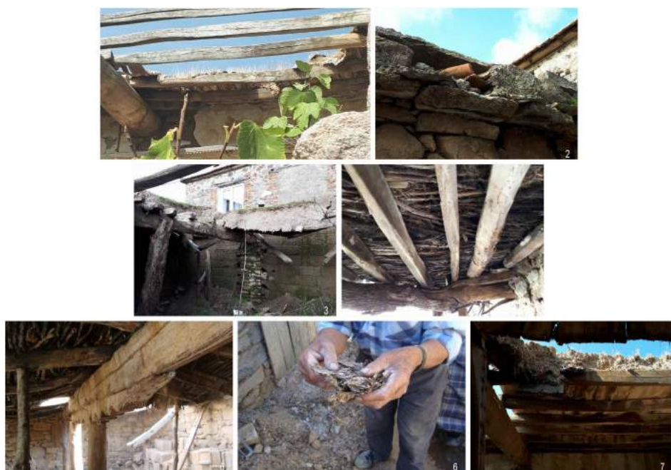
Figure 8. Traditional earthen flat roof elements. 1. Main beam, secondary beams, lath, moss, and earth layers (parcel 1360). 2. Water spout (parcel 1468). 3. Post, main beam, secondary beam, and earth layer (parcel 1468). 4. Secondary beams, branch, bush and moss layers (parcel 1468). 5. Post, bolster, main beam, secondary beams, and sandalwoods as covering layer (parcel 1487). 6. Moss from the roof in the hands of Koşfur (parcel 1487). 7. Main beam, secondary beams, earth layer (parcel 1497).
