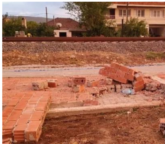
Figure 2. 8. The collapsed independent wall in Aydın (Source: Türkiye Gazetesi 2021)
