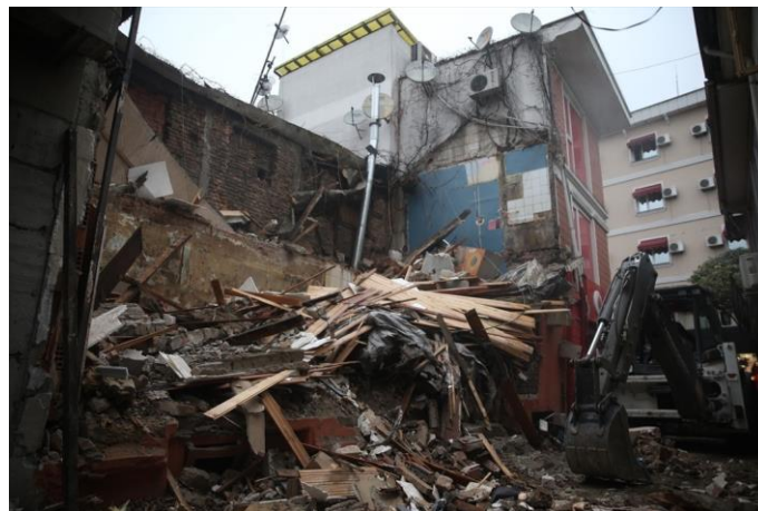
Figure 2. 10. Small earth mover used in a narrow Street in Düzce (Source: Haber 1 2022)
