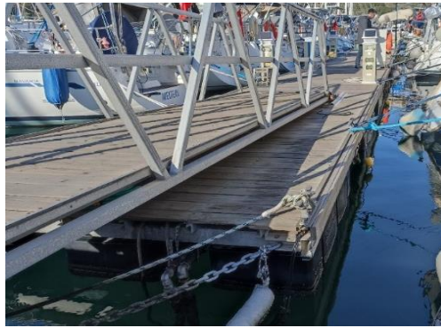
Figure 3.10. Gangway and connection chain between the quay and a floating pontoon.
