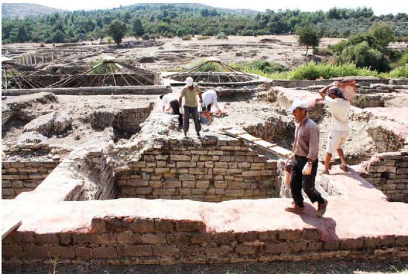
Figure 9. Photograph of capping of the ancient walls (IZTEK 2010, December) (color figure available online).
