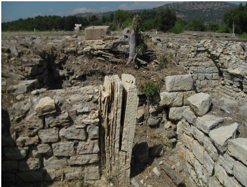
Figure 3. Photograph of conservation problems in the exposed archaeological structures (June 2010) (color figure available online).
