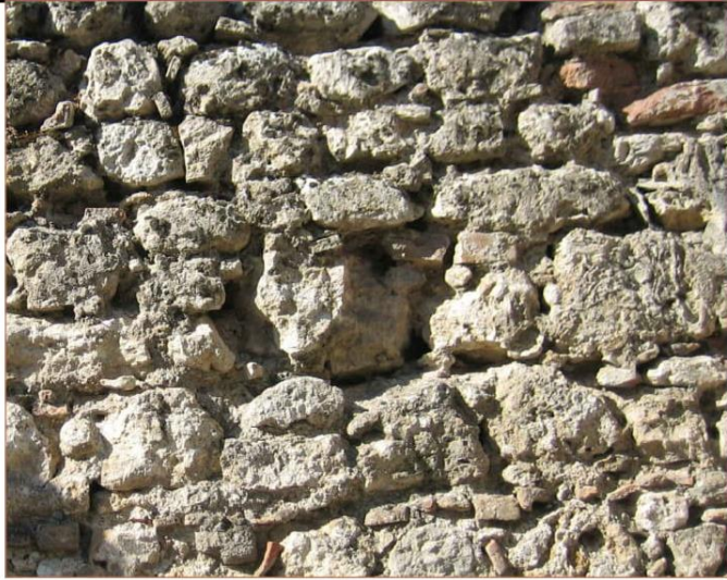
a. Load bearing wall: Rough cut stone at both surfaces, rubble stone and lime mortar in between
