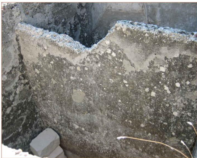
c. Non-load bearing walls: Cement interventions
