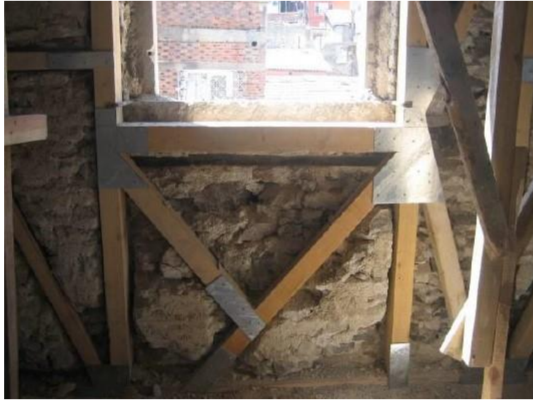
Figure 2.25. Strengthening of the wall with stainless steel bolted galvanized chrome nickel connection elements (Source: İpekoğlu et al, 2014)
