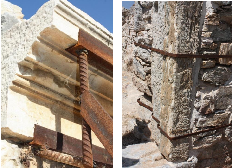
Figure 2.23. Rusting problem in a Roman (left) and Byzantine (right) ruin (Source: Turan, 2018)
